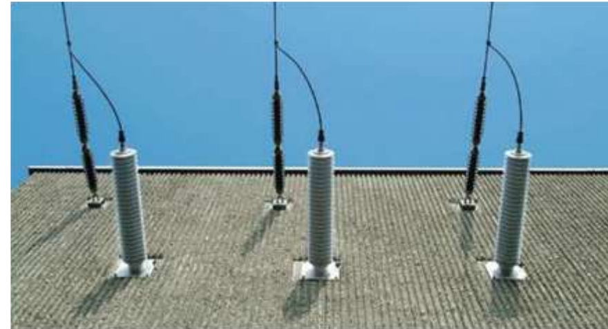
Wall & Transformer Bushings
